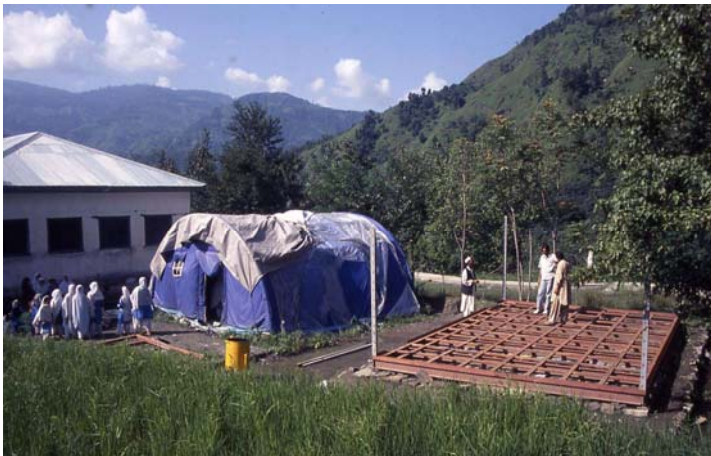
Old, temporary and new school being rebuilt following earthquake in Pakistan. Photograph by Andrew Hall
